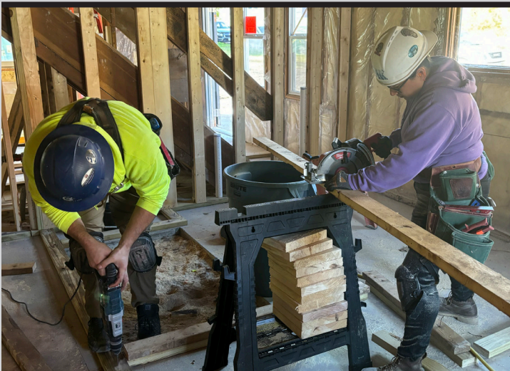
Two fourth-year apprentices from CTI Twin Cities Campus preparing framing for the main level.
