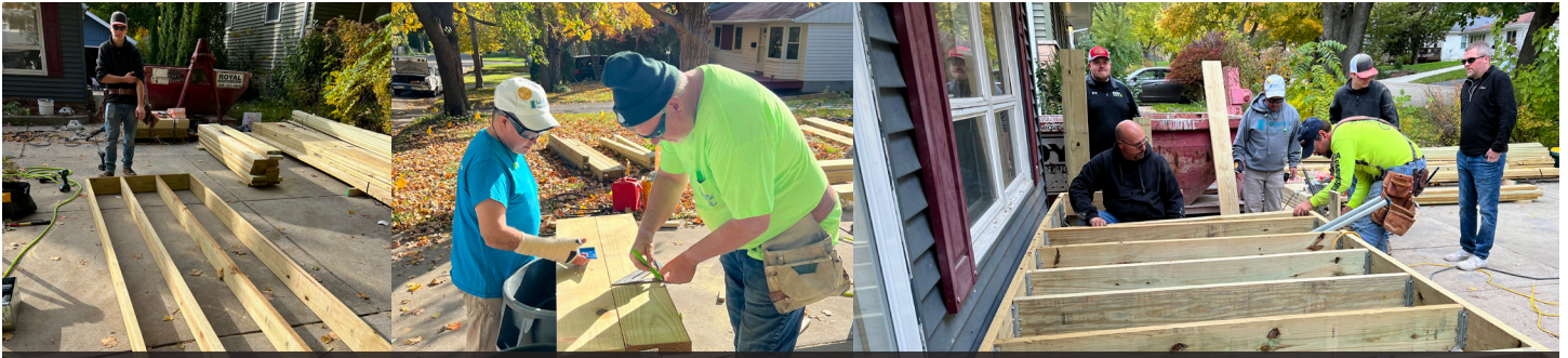
Photos left to right: Local 314 apprentice Cal Conway with a section of the ramp he framed; Local 314 Business Representative Scott Watson (R) and Joe Herr, founder of Logan's Heart & Smiles, measure and marking some boards for the ramp; Local 314 Business Representative Mike Higgins (L) and Apprentice Josh Dodge (R - in Hi-Vis) work on framing some stairs at the end of the framed platform.
