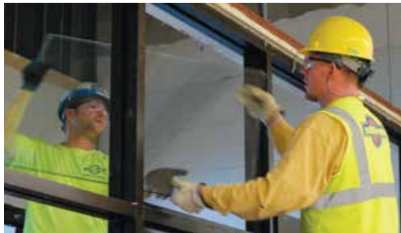
At left, Eric Thomma, Local 955, of Miron Construction works with a laborer in the demolition of a former Green Bay Cub Foods, which is being transformed into a Burlington Coat Factory store.
