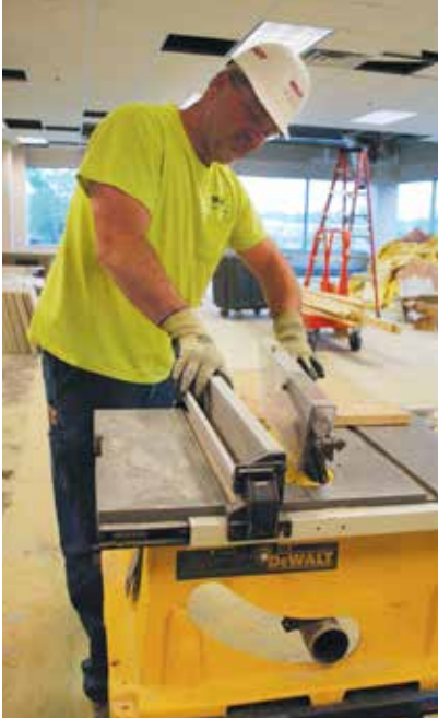
Blaine Brunette, Local 1146, working at Two Neenah Center in Neenah, Wis. Working for The Boldt Company, he is renovating a second floor for telemarketing firm Alta Resources.
