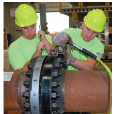
Millwright Local 1056 apprentices Sam Hilgart and Nick Hoffman tighten a flange with a hydraulic tensioning system.
