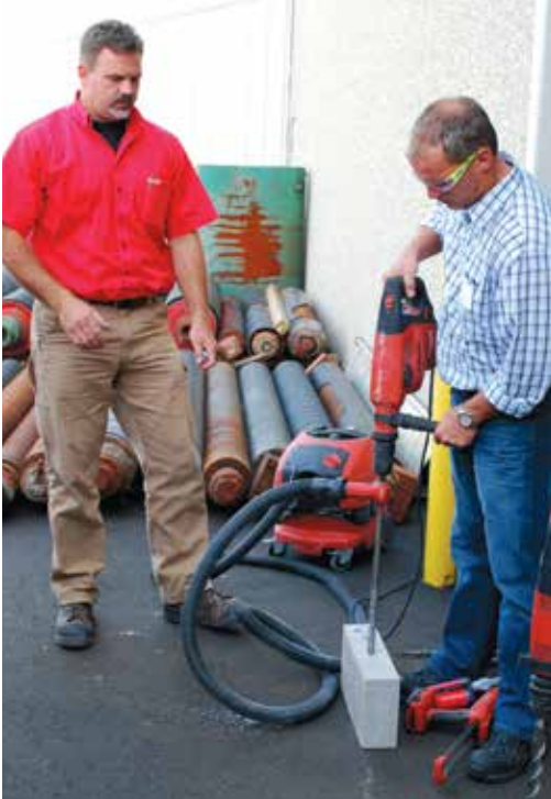
Dan Frase of Hilti, left, demonstrates a hammer drill bit that vacuums while drilling to Shane Hoffman, Local 1056, of Miron Construction.
