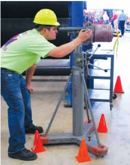
Millwright Local 1056 apprentice Jordon Fellenz shoots optical alignment with a precision level.
