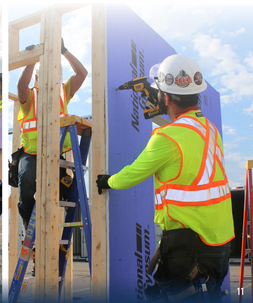
Jorge Rivera (left) and Juan Aguilar (right) framing walls and hanging drywall.
