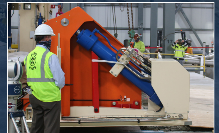
The last piece of mill equipment, the rewinder section of the new mill, is set into place during the stack-out at Green Bay Packaging.
