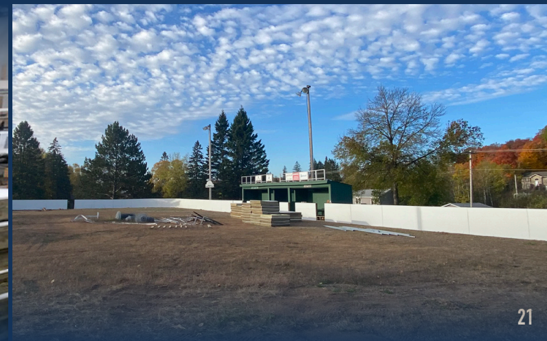
Duluth Heights Park hockey rink during the two-week reconstruction by Duluth apprentices.
