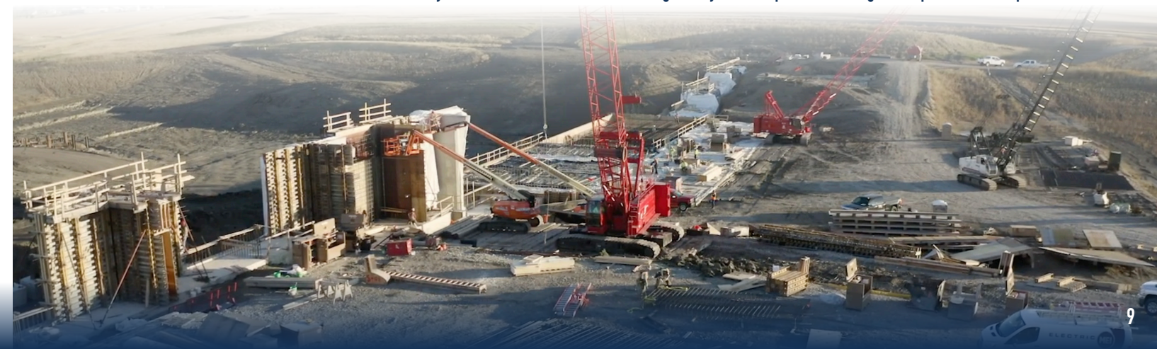
A bird's-eye view of the Red River structure being built by union carpenters, millwrights and piledrivers in September 2020.
