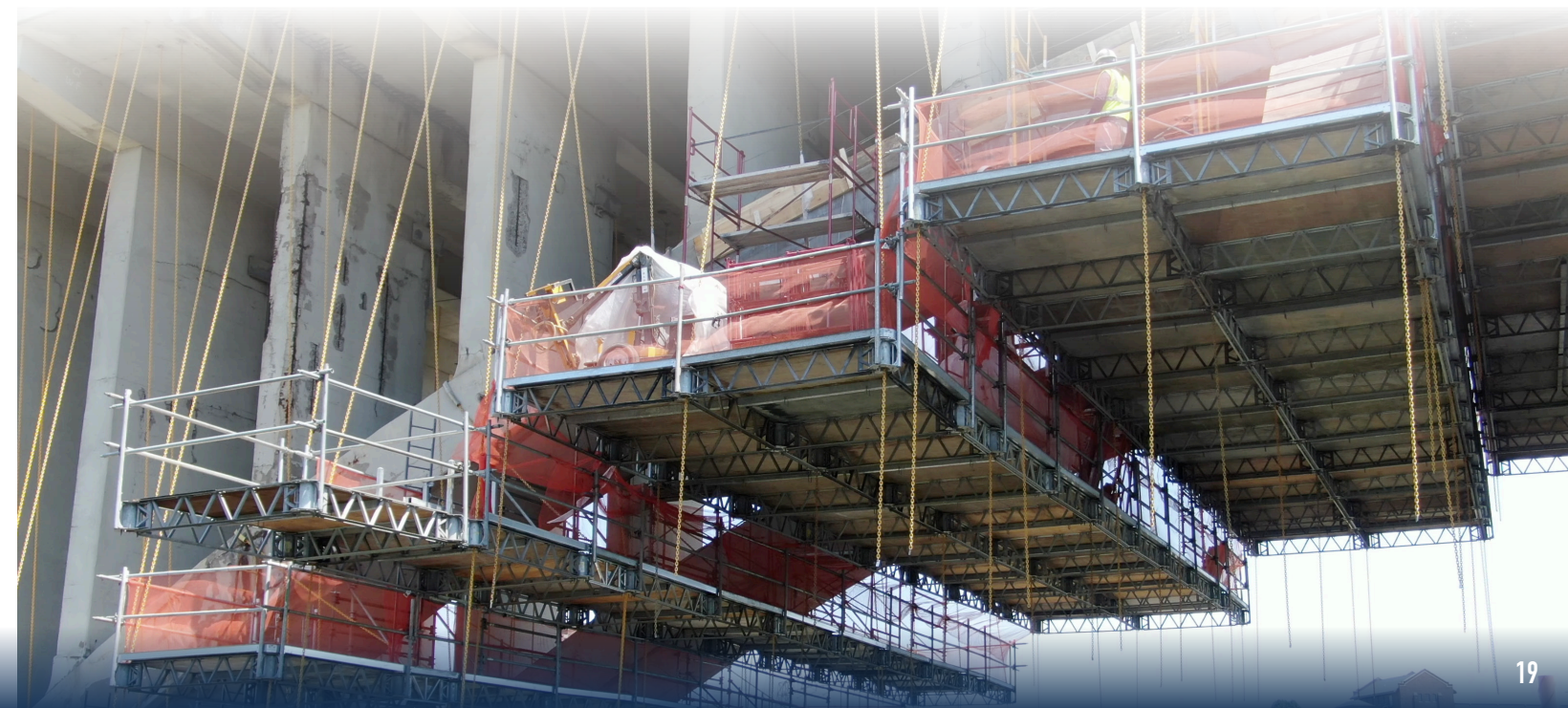
The BrandSafway's Quikdeck system allows carpenters the ability to safely work on an open air, modular platform. It can be configured into different shapes and sizes to accommodate the work that needs to be done on difficult to reach places like concrete arch bridges.
