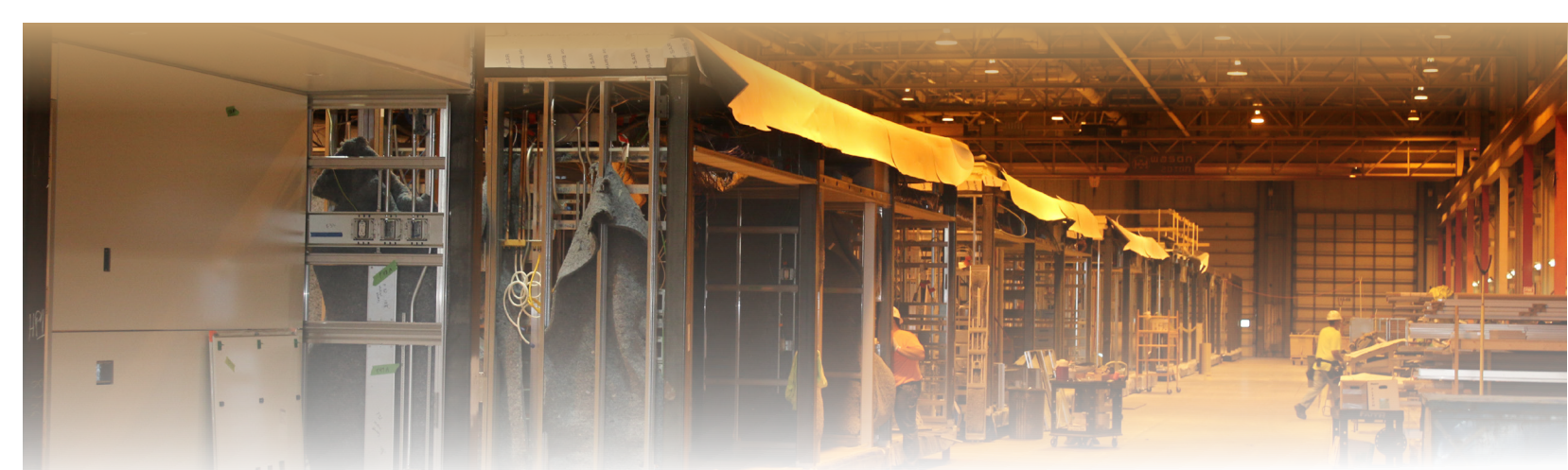
Prefabricated intensive care unit pods being built in Wisconsin and shipped to Georgia.
