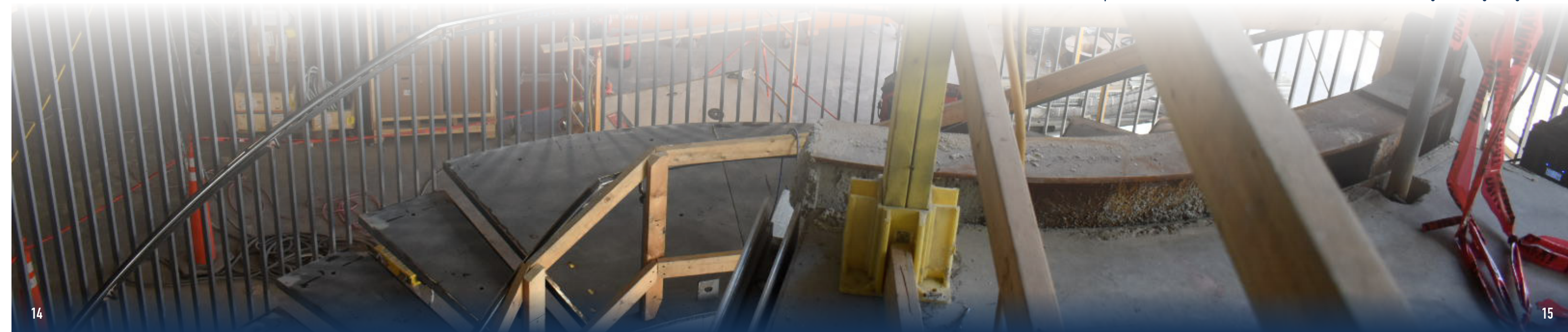
A new spiral staircase in the addition from the first to the second floor ballroom for weddings and other gatherings.
