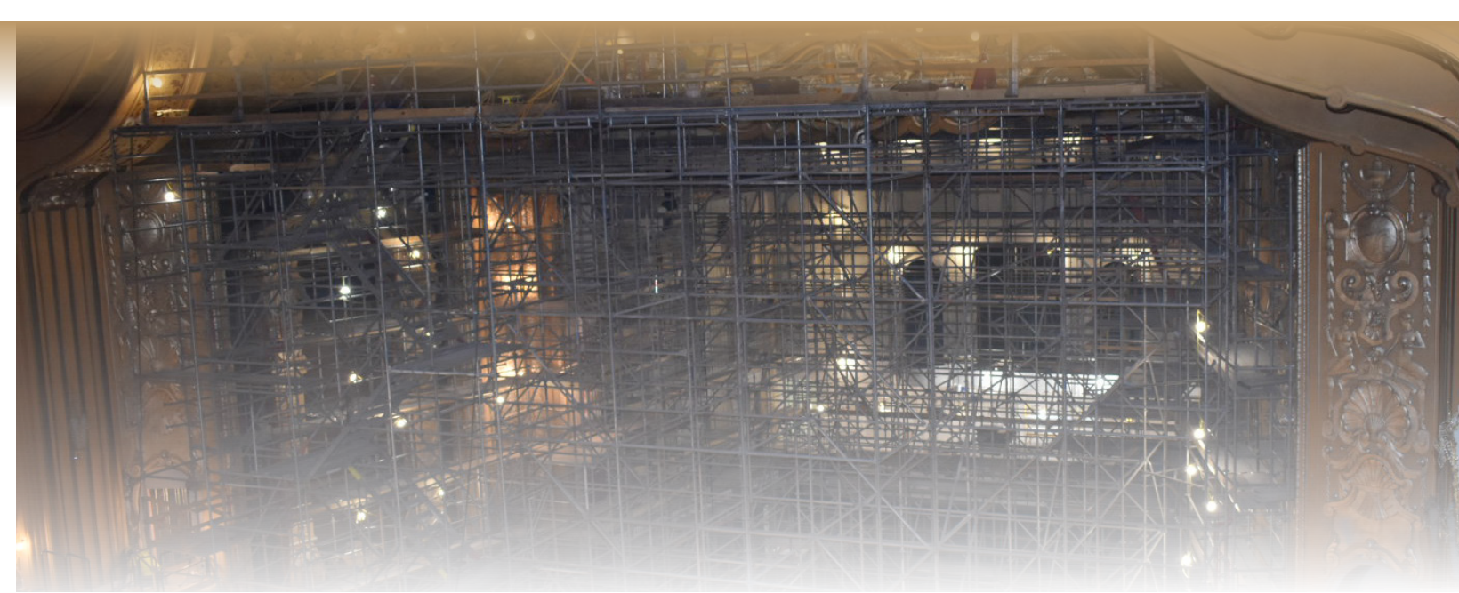
Complex scaffolding inside the newly coined Bradley Symphony Center during renovations and restorations.
