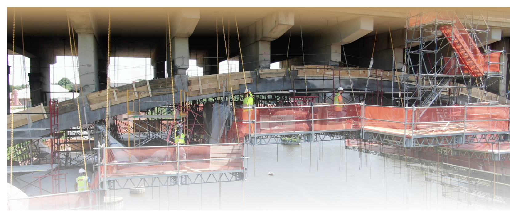
Carpenters working on the Tenth Avenue/Cedar Avenue bridge using BrandSafway's Quikdeck system.
