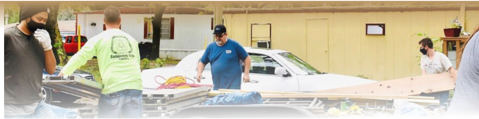
Students from the University of Iowa and local carpenters volunteered for the weekend to help repair the Forest View Homes. Supplies and materials were paid for by Iowa City.
