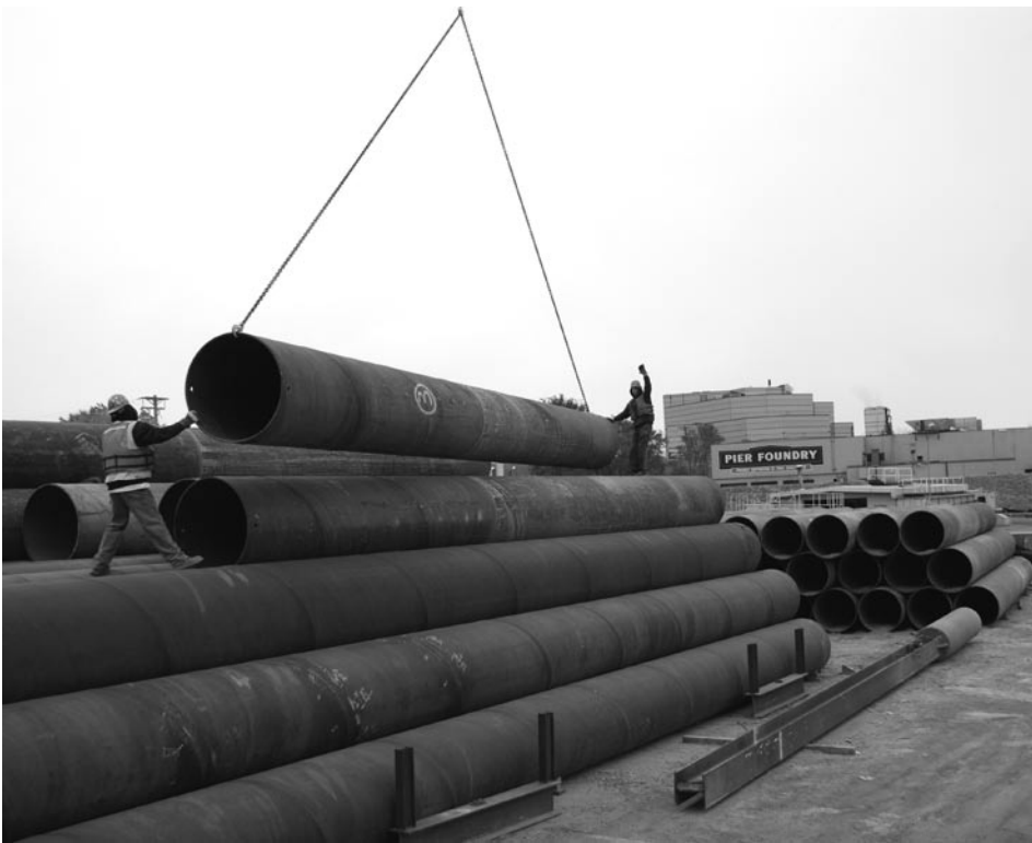
Mike Fetzer, Local 322, and Joe Lahr, Local 1847, stack 42-inch heavy wall piling.
