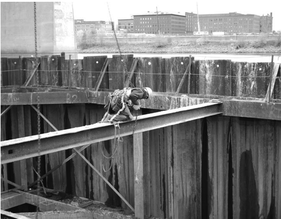
Paul Langer, Local 1382, removing the center strut in the coffer dam so structural columns for the northbound bridge can be poured.
