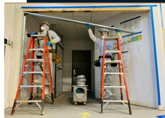
Top: Nick Gant and Porcha Shadd (both Local 361) tape off a wall opening. Middle: Tyler Kemp (Local 606) and Shadd tape a filter onto a door opening. Bottom: Zach Sadenwasser (Local 361) and Austin Seidel (Local 2934) are erecting a softwall containment system.
