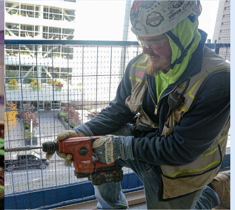
Frank Dolincheck V (Local 427 - Omaha, NE) hammer drilling cable barrier holes in parking ramp columns.
